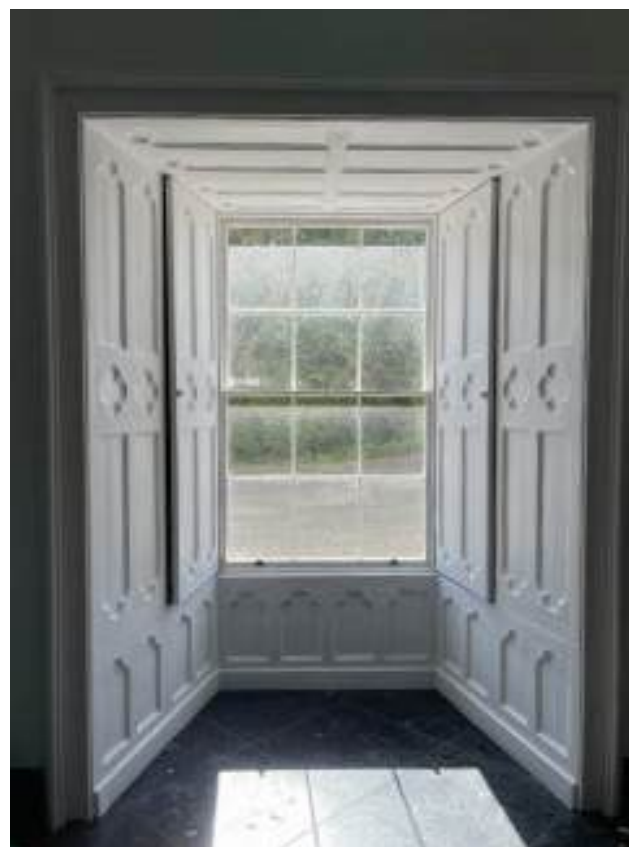
Front window on first floor of Áras na hOidhreachta prior to work carried out, 2025
