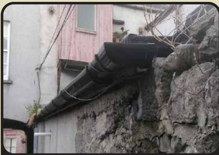
Clogged with vegetation at one end and with a clear gap at the other, this gutter is bringing water back into the building.
