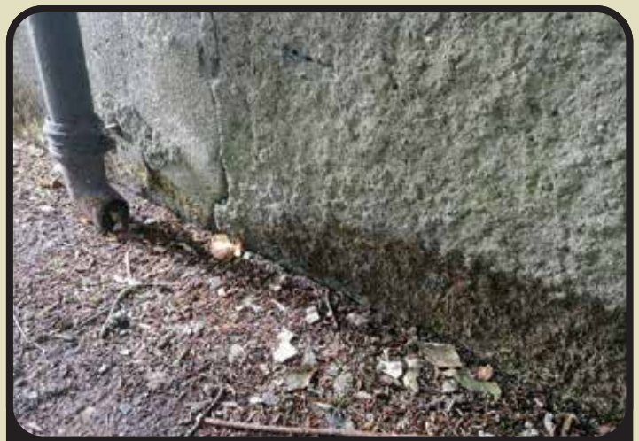
Water from this downpipe is being directed against a wall, causing it to be saturated.
